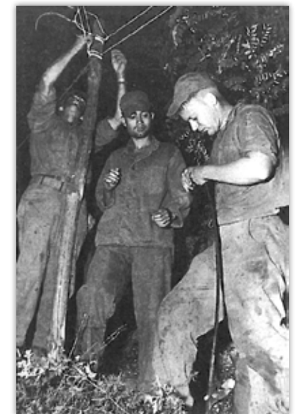
Navy Seabees (left to right) Electrician’s Mates Troy Edwards, Julian Perez, and Joseph D. Edson install floodlights on Red Beach at night on the 15th so that naval forces can sustain their critical over-the-shore logistics operations. (USN 420068)
