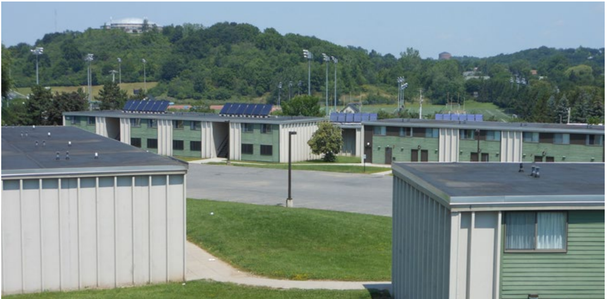
SOLAR PANELS INSTALLED ON THE ROOFS OF SOUTH CAMPUS TOWNHOUSES SUPPLY 50 PERCENT TO 60 PERCENT OF THE ENERGY NECESSARY TO HEAT THE WATER FOR THE RESIDENTIAL UNITS. ©2000-2015 ZACKIN PUBLICATIONS INC.
