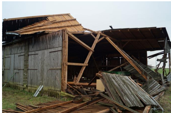
Figure 5. Damage to a shed in Barenthin, Germany on 10 November 2017. Photo: Thilo Kühne.
