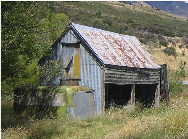
very weak frame with metal panels
