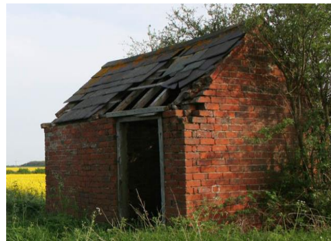
weakened brick wall structure
