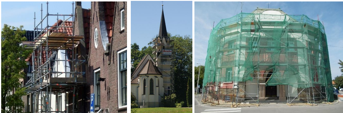
Figure 12. Scaffolding. Left: by Plaats - Own work, CC BY-SA 3.0, https://commons.wikimedia.org/w/index.php?curid=17360293 Centre: by TheRunnerUp - Own work, CC BY-SA 3.0 at, https://commons.wikimedia.org/w/index.php?curid=28131152 Right: by Globetrotter19 - Own work, CC BY-SA 3.0, https://commons.wikimedia.org/w/index.php?curid=44053732
