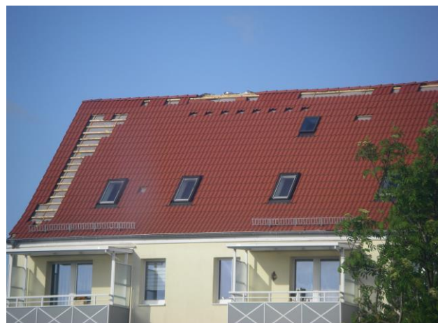
Figure 7. A roof with a number of tiles having blown off in Bützow, Germany. Photo: Thilo Kühne (ESSL).
