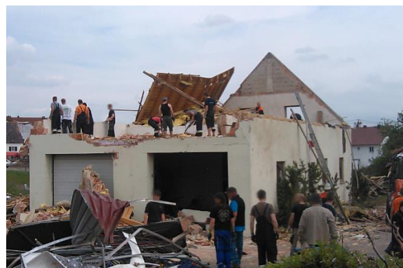
Figure 6. House deroofed by a tornado in Affing, Germany on 13 May 2015. Photo: Pieter Groenemeijer (ESSL).
