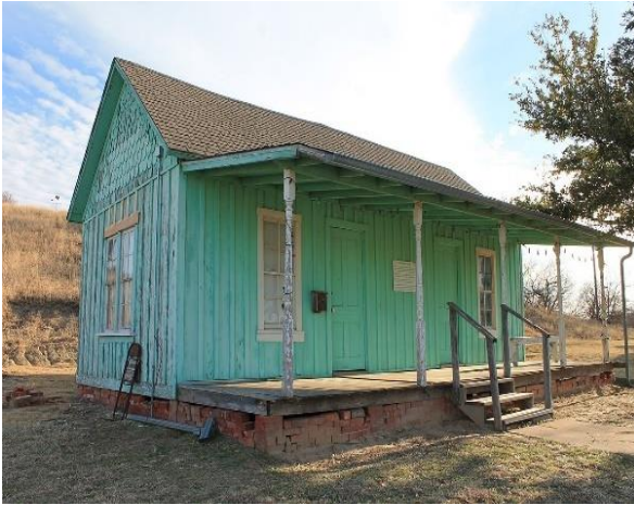
weak wooden frame with wooden panels
