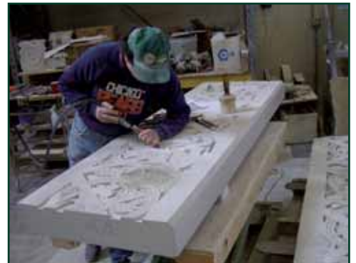
Walter Arnold perfects the ornate details of the limestone friezes which will replace damaged pieces above the Jackson Street sidewalk.
