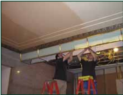
Electricians finish the wiring on the renovated lighting fixtures in the lobby.
