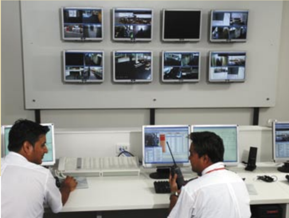
The control room for the new Woolworths' integrated security system.
