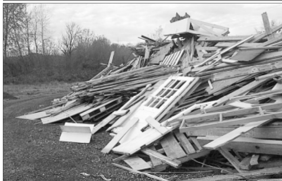
LOOKS LIKE MULCH: This wood debris is destined for mulch. About 18 to 20 tons of wood chips are produced from wood waste every time the wood grinder visits campus.
