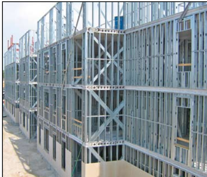
Figure 1: A 4-story building using CFS stud walls supporting precast hollow core concrete planks
