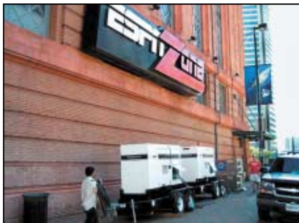
shown working outside the Hard Rock cafe. Above Center: Two 56-kW diesel generators rented by Trade-Winds Environmental to power drying equipment are shown in operation at ESPN Zone. A 200-kW generator was also utilized.
