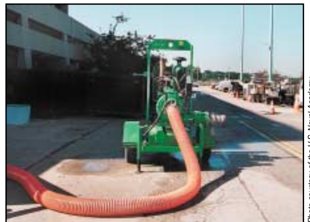
Above: A 6” diesel trash pump is shown in operation at the U.S. Naval Academy in Annapolis, MD. Whiting-Turner Contracting Co. rented this pump and a 12” Quiet Flow™ to pump out a flooded mechanical room on the campus.
