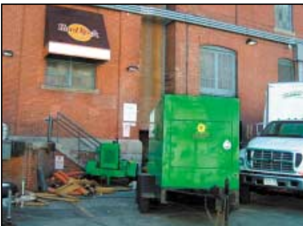
Baltimore’s Inner Harbor suffered extensive flooding and water damage from Hurricane Isabel’s storm surge. Above Left: Two diesel pumps, a 4” trash pump and an 8” Quiet Flow™, were rented by Rolyn Construction Corp. and are
