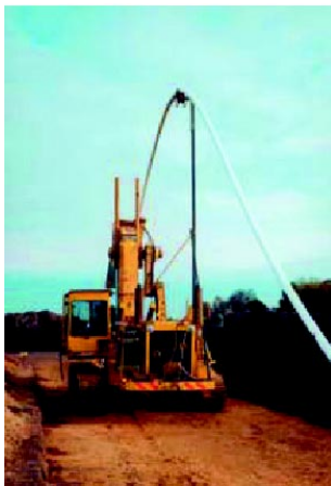
Figure 10 Installation of RTP by trenching machine at 1.5 m depth and a speed of 400m/hour
