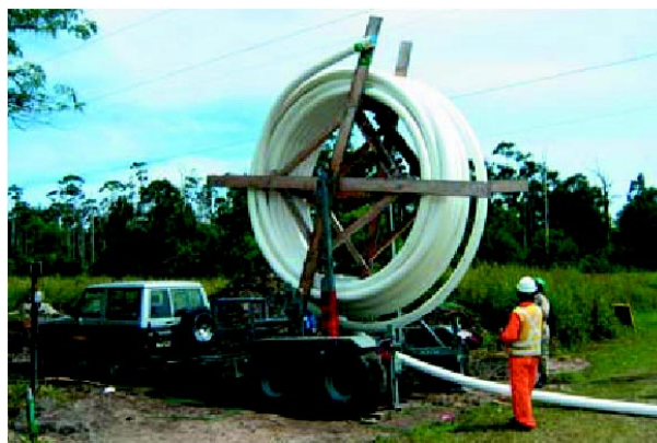
Figure 8 Uncoiling RTP from disposable wooden reel by simple installation trailer behind a 4WD vehicle.
