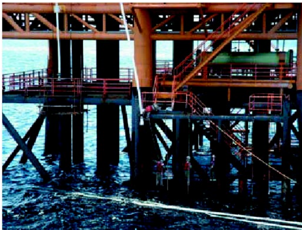
Figure 11 Installation of RTP water injection riser on a platform of BSP. (courtesy: Brunei Shell Petroleum)
