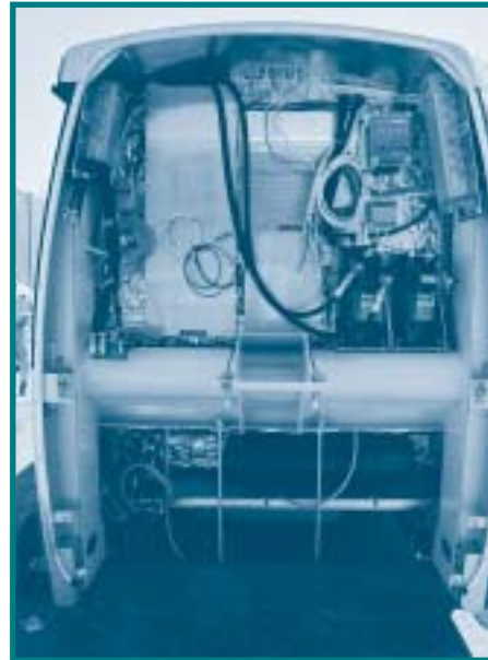
Project design/build contractor, Schwager Davis, inc. (SDI) performed wiring and final assembly of the Swiss-made trains in Indianapolis.
