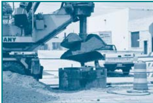
Foundations for the guideway columns of Clarian’s People Mover system were dug to an average depth of 27 feet.
