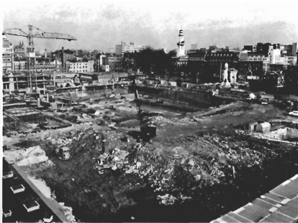
Both pictures show excavation work for reception and departure areas for cars and taxis
