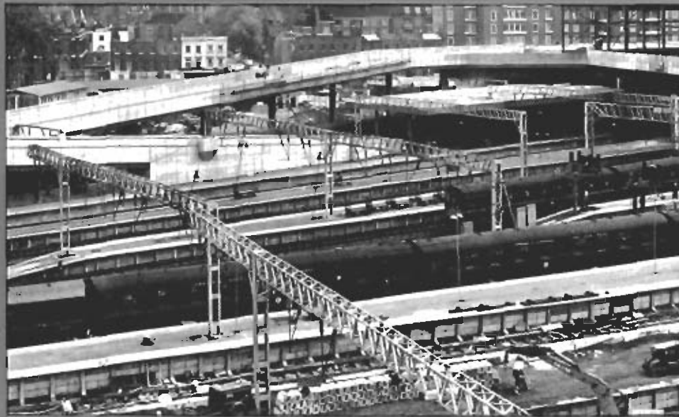
View of the platforms from the signal box, some of which are under construction, taken in May 1965
