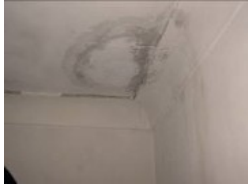
Water damage to ceiling of museum (detail)
