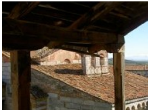
Damage to roof beams
