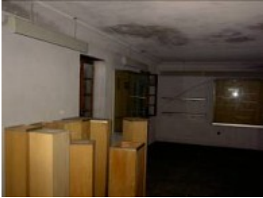
Water damage to ceiling of museum
