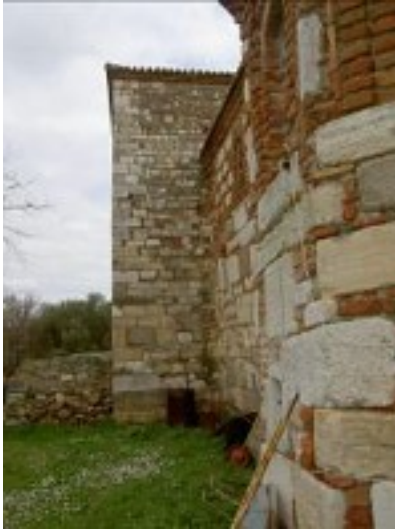
Damage to walls
