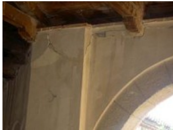
Damage to walls and roofing in statuary portico
