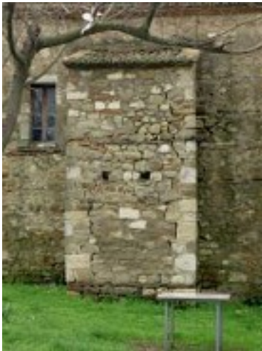
Damage to walls
