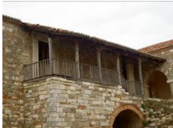
Damage to balcony woodwork
