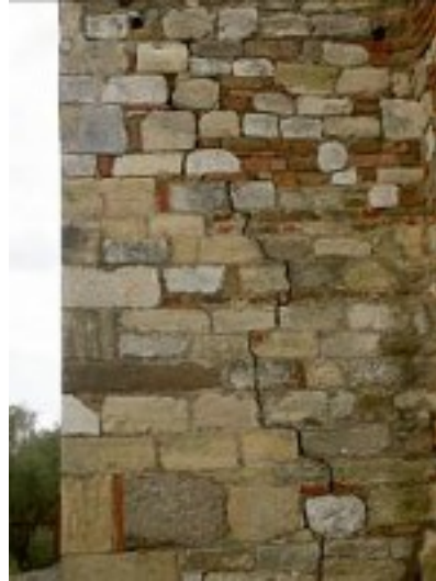
Damage to walls (detail)
