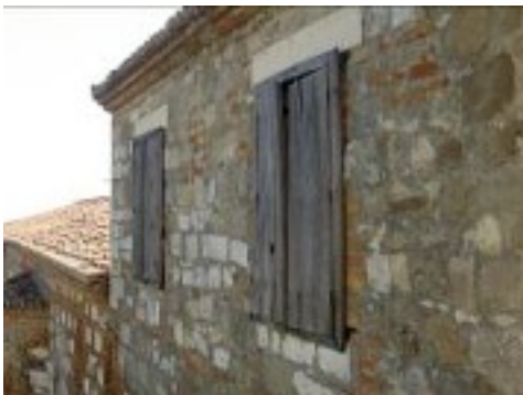
Damage to shutters
