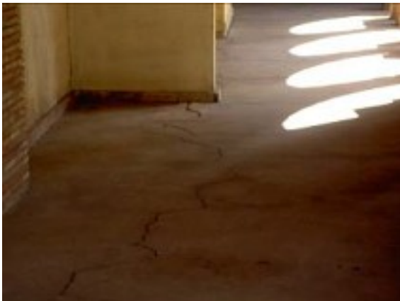
Cracks in floor of statuary portico (detail)
