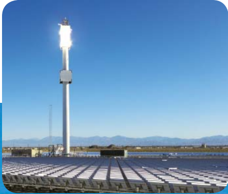
Solar thermal receiver
