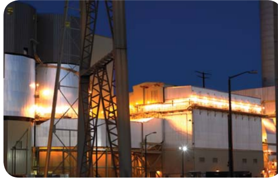
Multi-pollutant control systems
