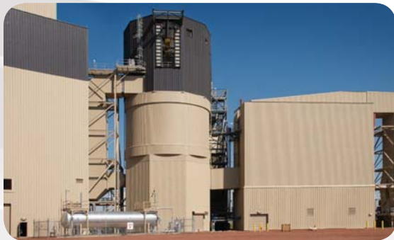
Dry flue gas desulfurization system and fabric filter particulate collection
