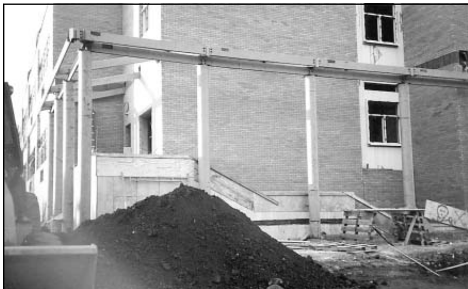
Brick by brick, Blind Brook Middle School nears completion as the school community busily prepares for the move in January. Photo by Mark Harris
