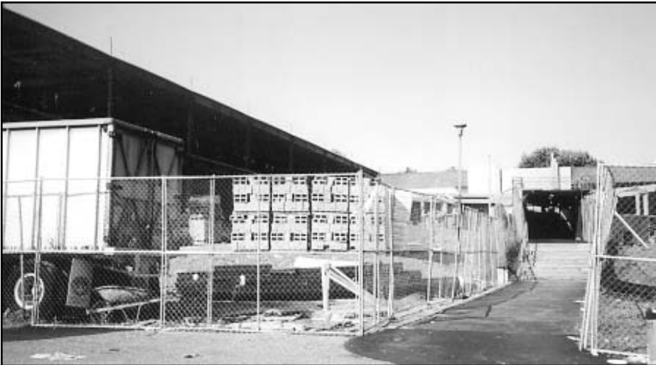
Blind Brook undergoes radical changes as the new Middle School takes shape. Photo by Mark Harris
