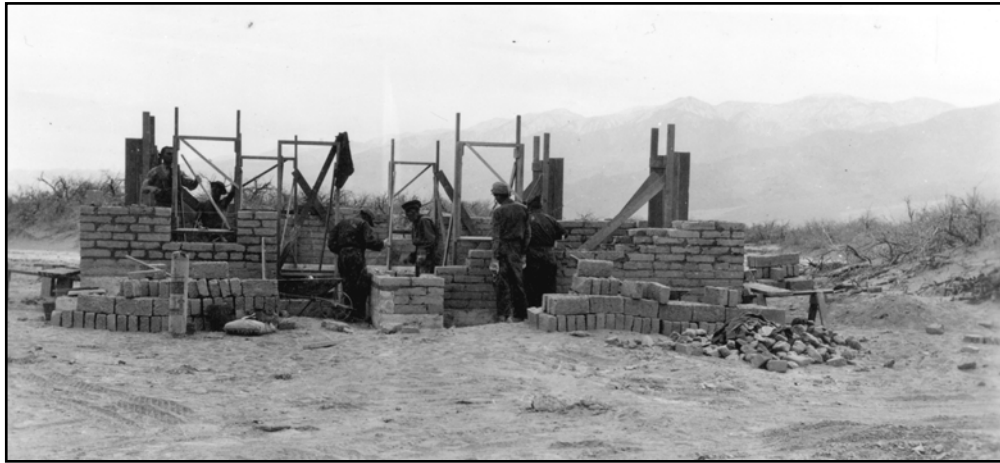
Photo 3. Adobe home for Timbisha Shoshone under construction by Civilian Conservation Corps, Furnace Creek, March 1937. Photo by John Bergen, Neg. No. 3275, Death Valley National Park Archives.
