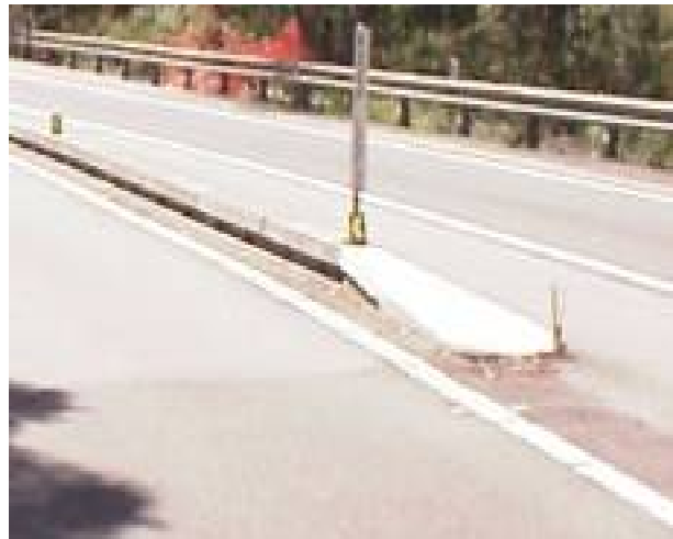
Elsholz redirective barrier
