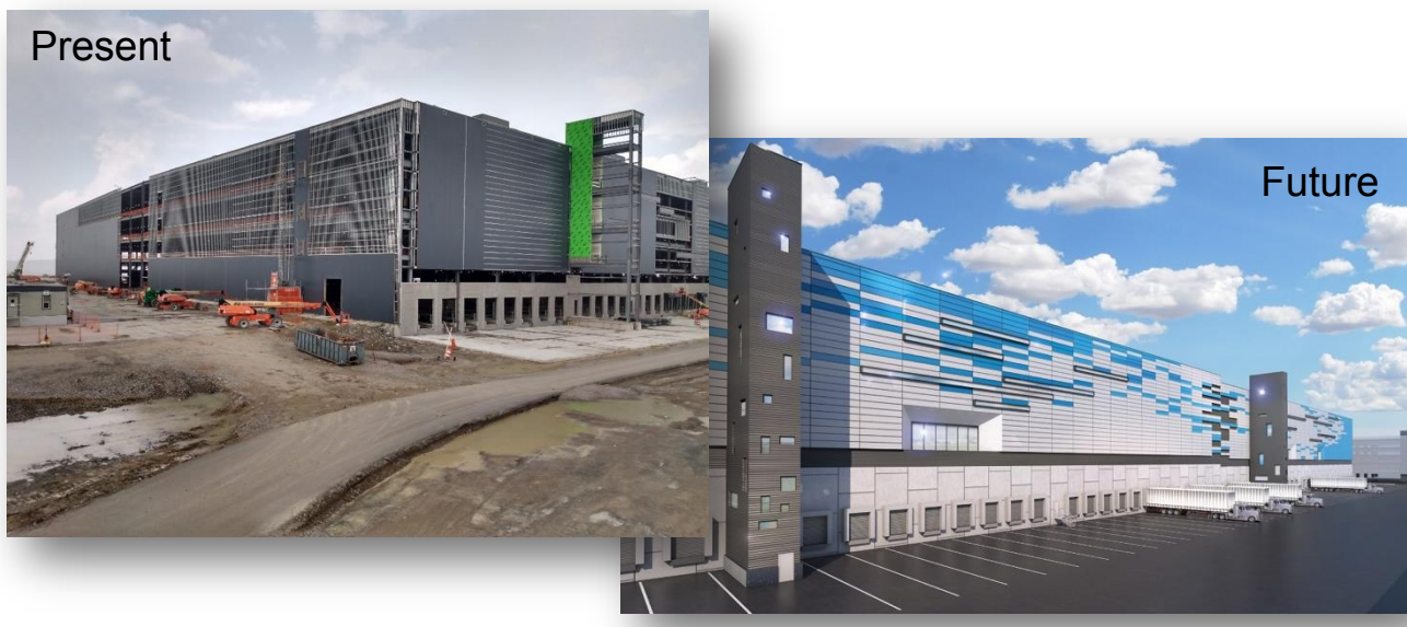
Amazon’s massive complex at Cincinnati CVG, pictured above on August 5, 2020, is in the final stage of construction. The airside portion of the structure is in the distance. Pictured at right is an Amazon-commissioned drawing of how the structure will look and how the truck bays will be used upon completion (left, Chaddick collection; right, Amazon).
