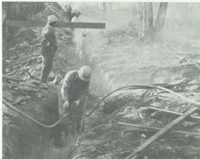
The Thin Grey Line as a sewer line goes through hard rock.
