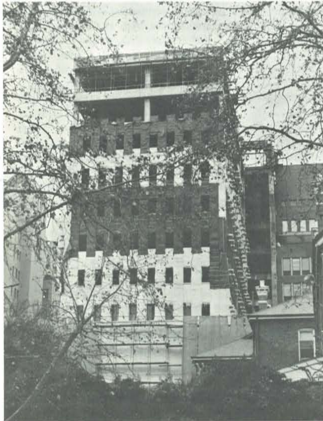
An artistic view of work in progress on the Reserve Bank project.
