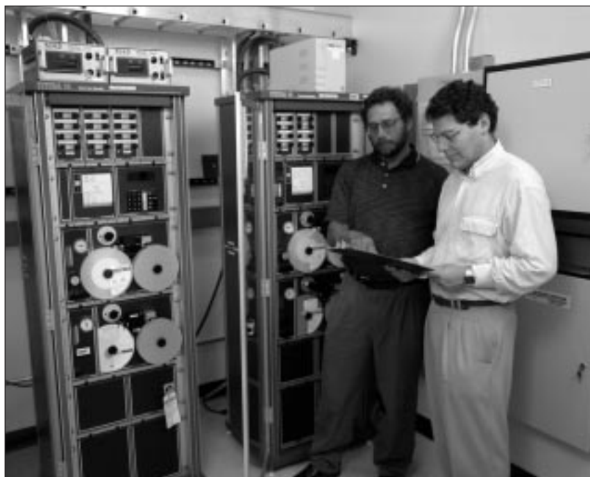
Paul Moskowitz and Ken Zweibel inspect gas-monitoring control panels at NREL’s Solar Energy Research Facility. Moskowitz is Division Head of BNL’s Environmental and Waste Technology Center; his PV credentials date back to 1978 when he was principal investigator for the lab’s PV Program. Zweibel, the Project Leader for the Thin Film PV Partnership, has authored two books on PV and has been involved with thin films at NREL since 1979.
