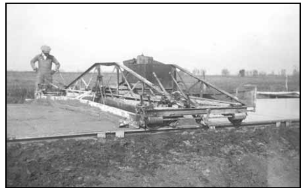
Concrete finisher on Highway 6 in Saunders County, c. 1921 (Photo courtesy of NDOR)
