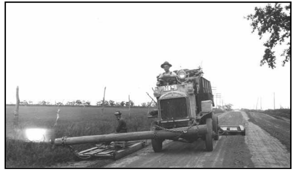
Equipment used to maintain a flat ditch near York, c. 1920s (Photo courtesy of NDOR)
