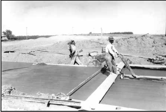
4.6-mile paving project in Scottsbluff County between Bayard and Scottsbluff in 1931 (Photo courtesy of NDOR)
