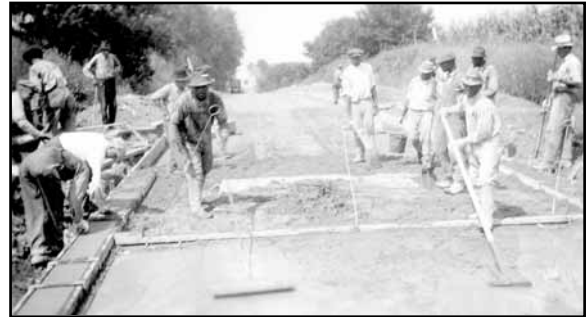
Laying concrete base for brick street near Elkhorn, Douglas County, c.1920 (Photo courtesy of NDOR)
