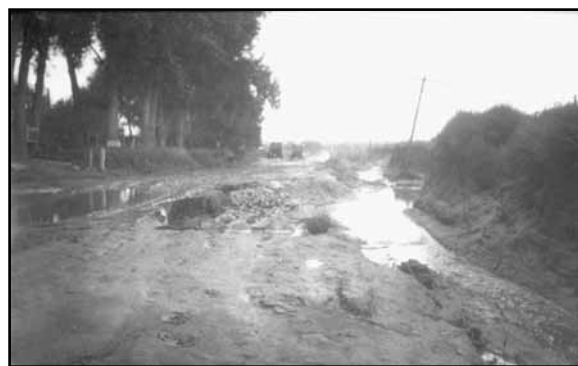
Example of poor drainage conditions of roadways (possibly in Red Willow County), c. 1925 (Photo courtesy of NDOR)
