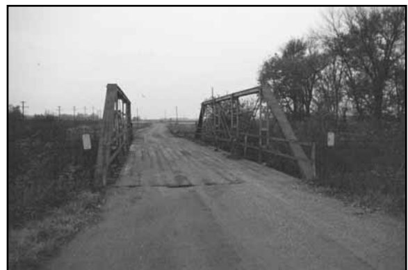
Pratt truss bridge, Duncan vicinity, PT00-145. Single-span, pin-connected structure is an early example of a bridge on the Lincoln Highway.
