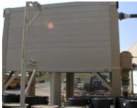
The new cooling tower system is one of the very few systems that is new and up to date. (Photo by Tammi Verhoeff)
