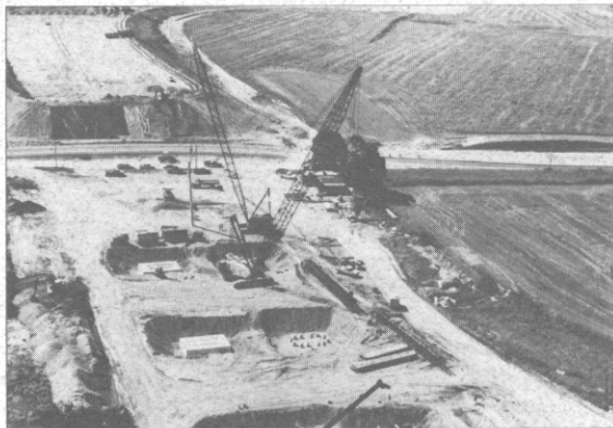
Piles and footings are the first concrete evidence of the new C&D Canal bridge, now well underway.
