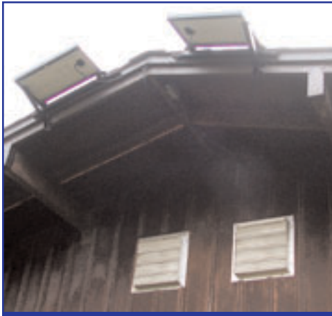
Portable classroom with PV panels on the roof and fan vents on the outside.
