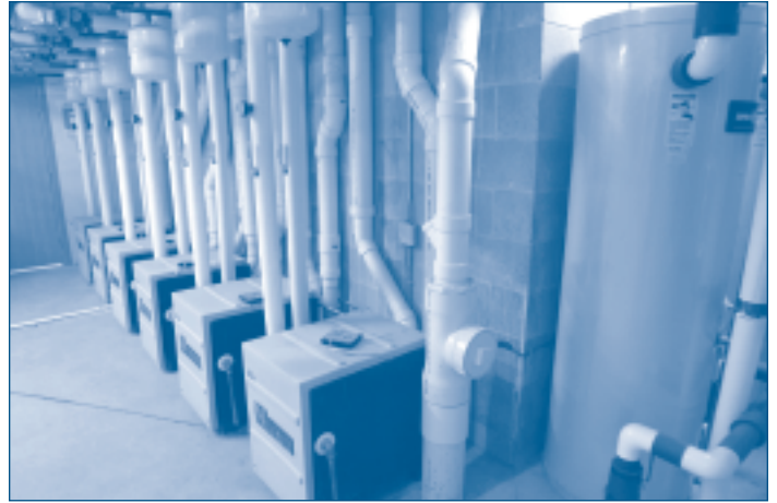
Six condensing boilers are installed in a Madison, WI, apartment building. Two of the boilers are dedicated to water heating and tied to big water tanks.
