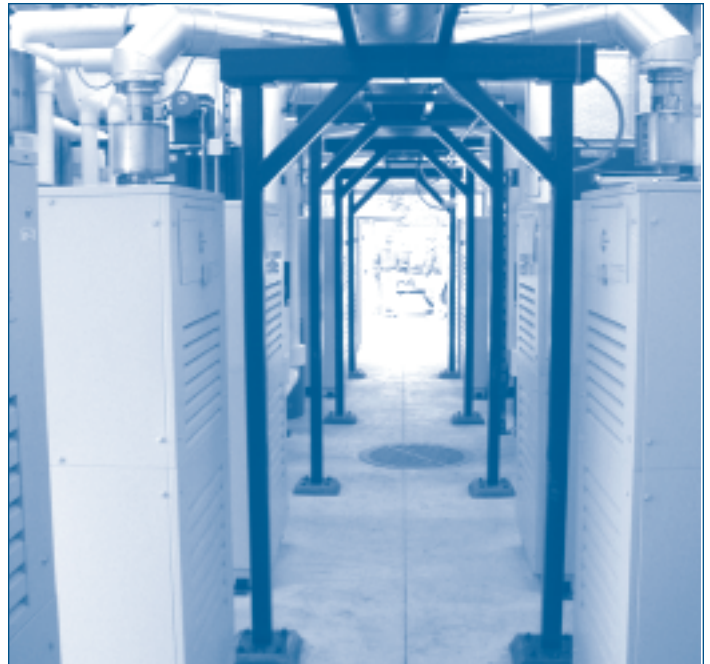
The set of microturbines at an Antioch, IL, high school, using landfill gas.
