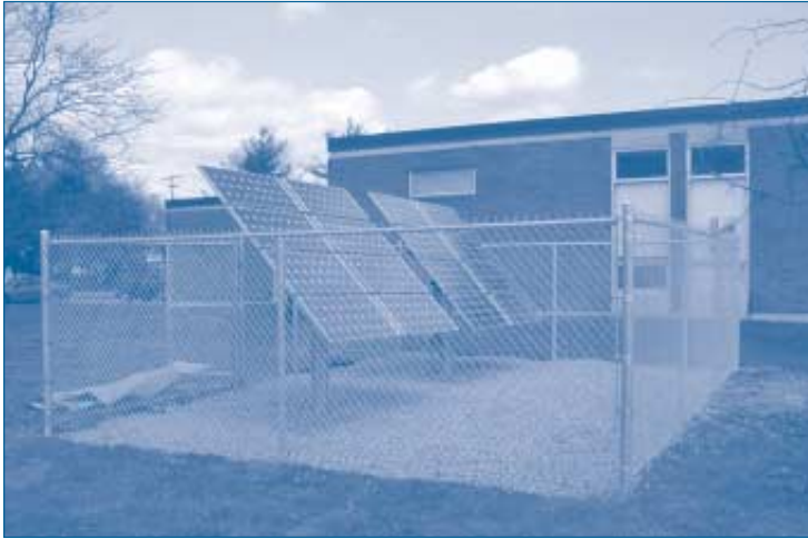
Photovoltaic panel arrays at Worthingway Middle School in Worthington, OH.
