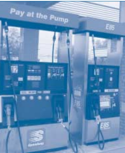
The first E85 Pump was installed at the Speedway gasoline station in Hilliard, OH.
