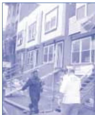
Work in the Building on Faith Blitz Build in New York City
