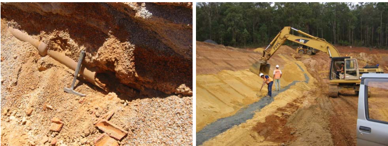
Figure 3: Waroona Dam – Photograph on left showing blockage of the old GEW drainage pipes and the high degree of contamination of the coarse filter media surrounding the pipes. Photograph on the right shows the construction of sandwich chimney filter system consisting of coarse aggregate sandwiched between sand at Waroona Dam in 2002.
