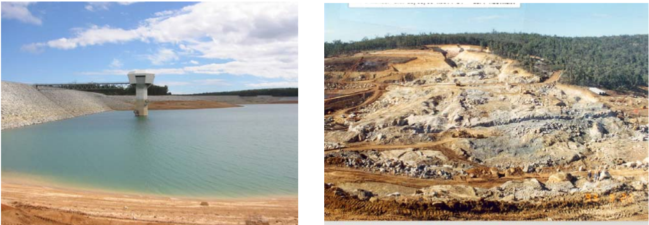
Figure 7: North Dandalup Dam, the corestones on the left abutment (see photograph on the right) caused considerable difficulty in preparing the foundation for the earth core and the rockfill zones of the embankment.
