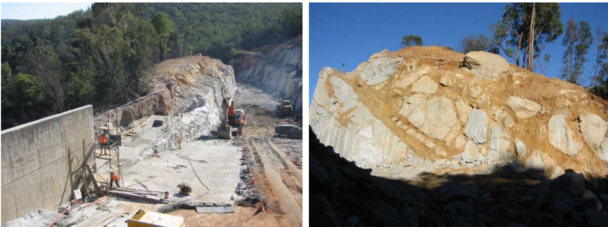
Figure 2: Serpentine Dam – Deepening of the spillway chute (2002) shown on the photograph on the left. The original invert of the unlined chute was at the level of the berm on the left hand side of the photograph. The photograph on the right shows the granite weathering profile. The original floor of the spillway chute was at the top of the cutting on the left of this photograph.
