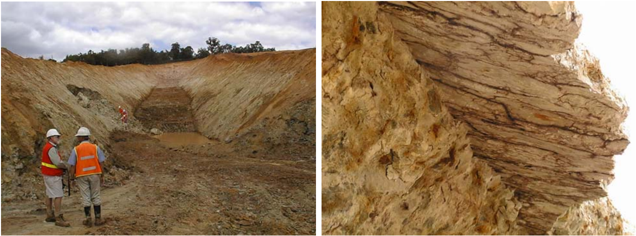
Figure 5: Cut-off trench through upper conglomerate at Harvey Dam (2001), photograph on left showing failure of sidewall along bedding plane surface and steeply dipping joint. Photograph on right showing underside of bedding plane surface.
