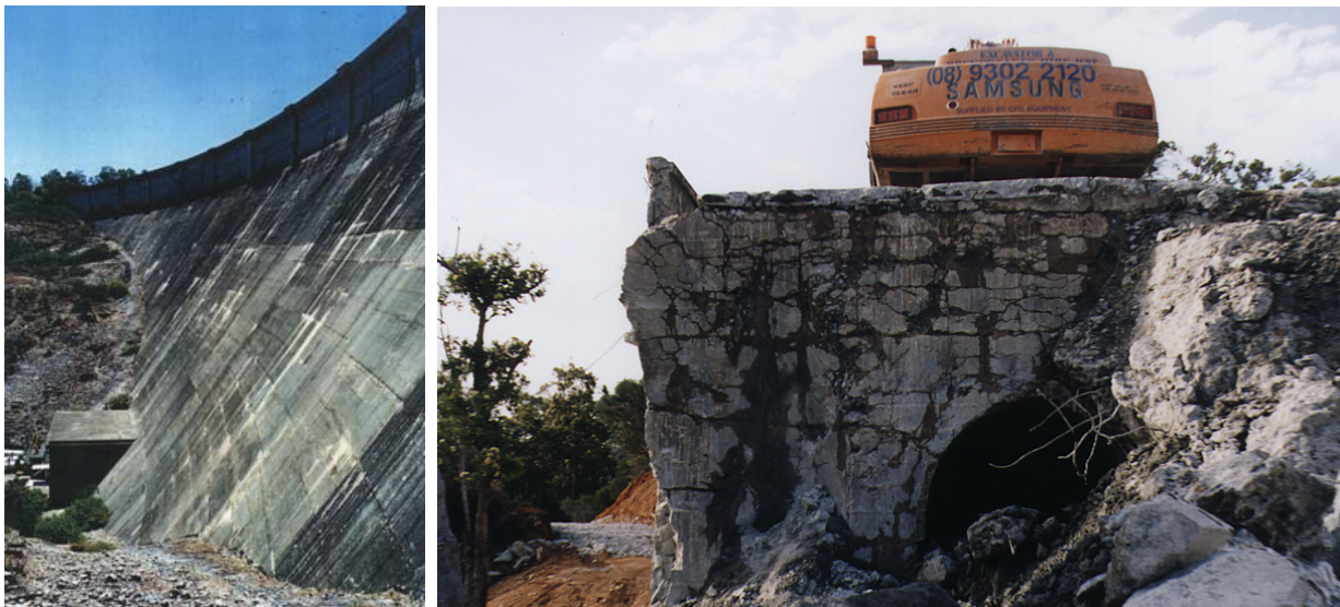
Figure 8: Canning Dam, the photograph on the right shows the extensive cracking in the region of the upper gallery, believed to have been caused by AAR.
