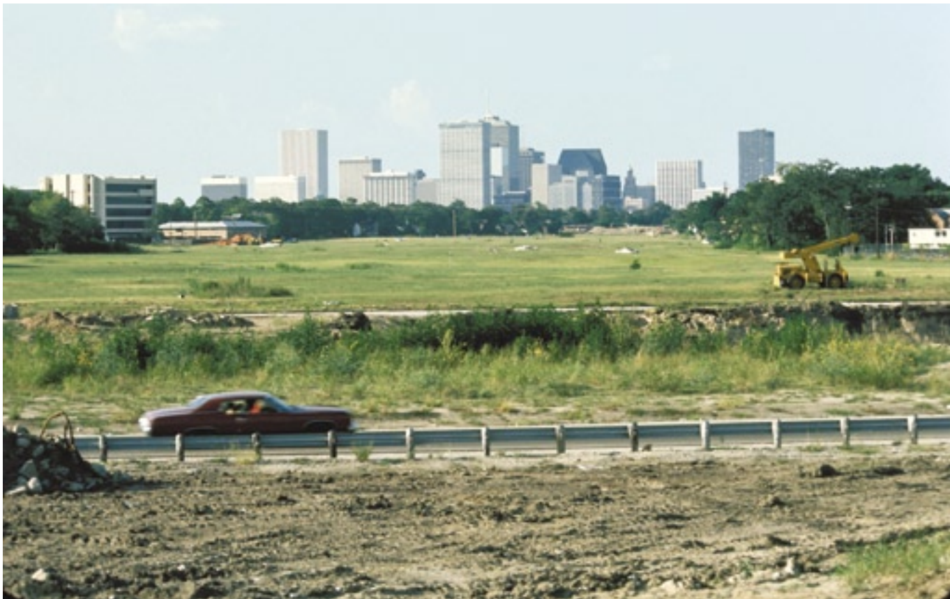
Freeway construction in slow motion: This September 1976 photo shows the cleared right-of-way corridor north of Brays Bayou. Right-of-way clearance began in the late 1960s and was complete by 1972, but the corridor sat vacant for more than five years due to funding shortfalls at TxDOT. The existence of such a wide corridor of clear land so close to the central business district for most of the 1970s was a remarkable novelty and is something that will probably never again be seen in any city in the United States in the context of freeway construction. (Photo: Chuck Fuhs)
