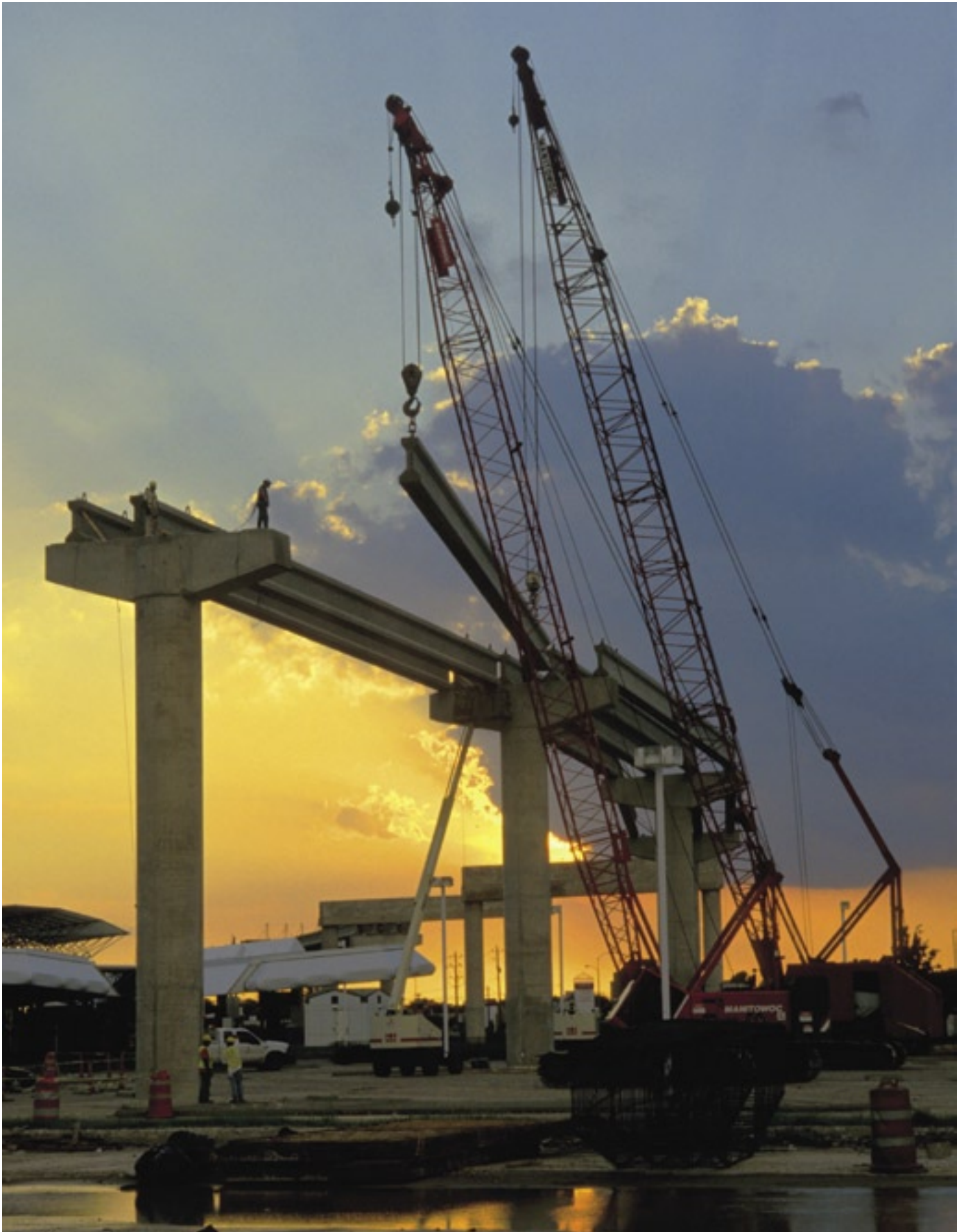
Beam placement: This view shows construction of the connector ramp from the Westpark Tollway to the Southwest Freeway, July 23, 2002.
