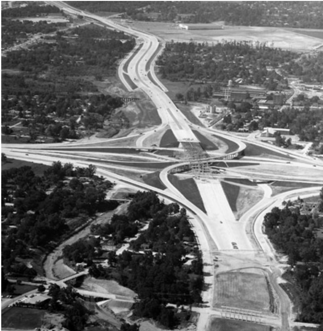
Loop 610 interchange construction: This view looks north at the three-level interchange with the North Loop in May 1961. The North Freeway north of Loop 610 had opened a month earlier, and the interchange was partially open to traffic. The North Freeway and the full interchange were opened in July 1962. (Photo: TxDOT)
