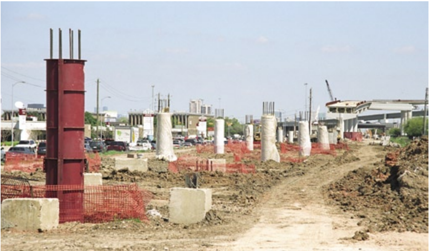
Westpark Tollway construction: This view looks east toward the Southwest Freeway interchange in March 2003.
