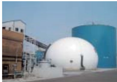
Chiba Biogas Center
