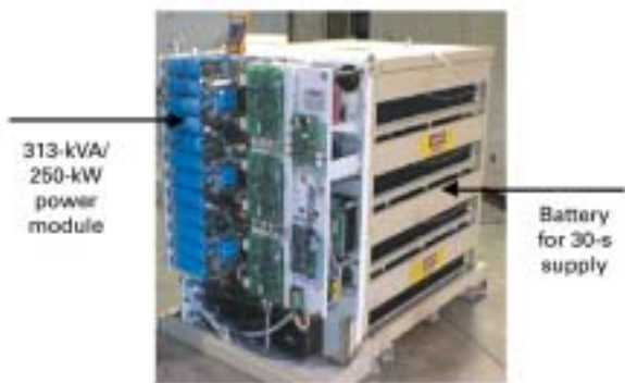
Exhibit 7.5 UPS module at STMicroelectronics, Phoenix, AZ (source: ESA/S&C PureWave)
