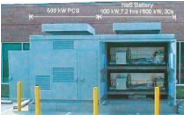
Exhibit 7.10 Na-S BESS supplying AEP offices in Ohio (source: ESA/NGK)
