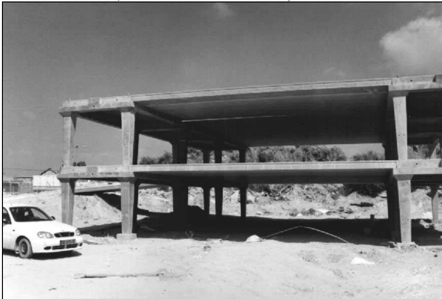
Figure 3: A full size structure of a parking lot at erection (design: Villa Nir, structure: Moshe Peer, construction: Solel Boneh).
