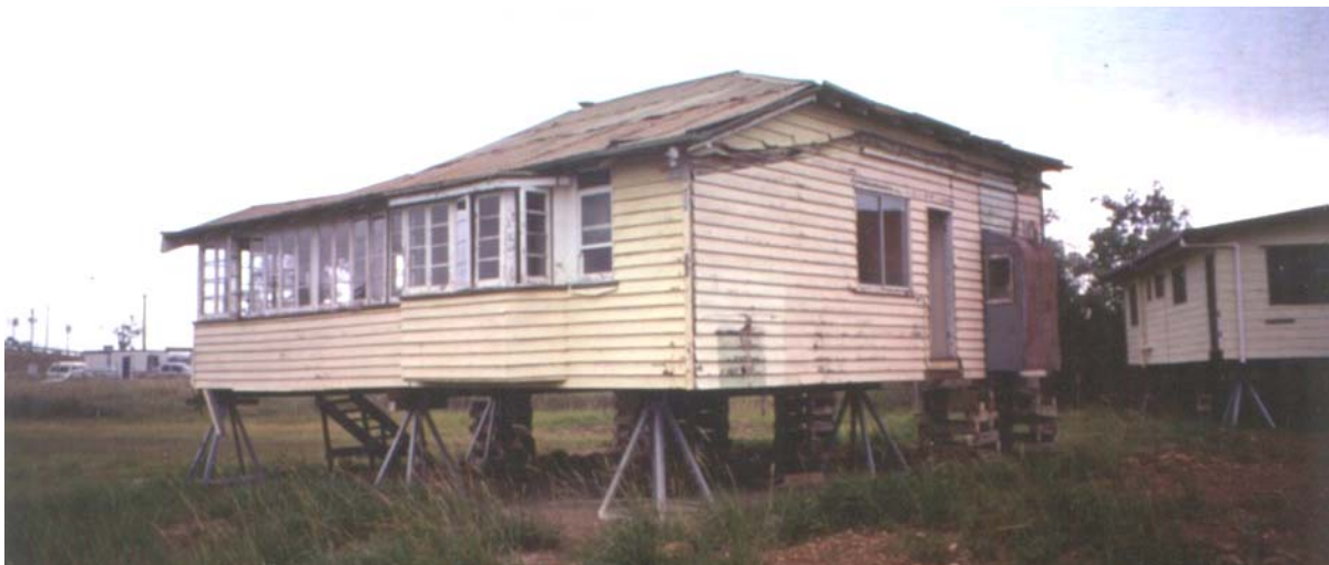
Figure 1 Typical timber house built in 1920's, now derelict and awaiting relocation or deconstruction for materials recycling.
