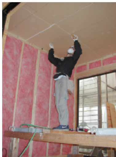
Photo 11 Ceiling gypsum boards hanged by metal connectors. Insulation fixed without using staples.
