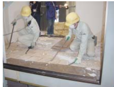
Figure 2. Removal of the flooring (Current design) – Floorings are removed by using deconstruction tools. Wood pieces and adhesive remains on the floor sheathings.
