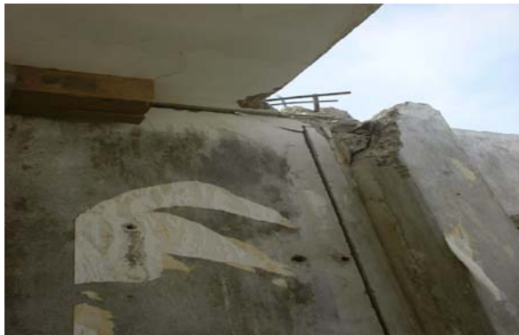
Fig 4: The newly settlement of the construction after sawing the wall in two sections. The right section will be removed.
