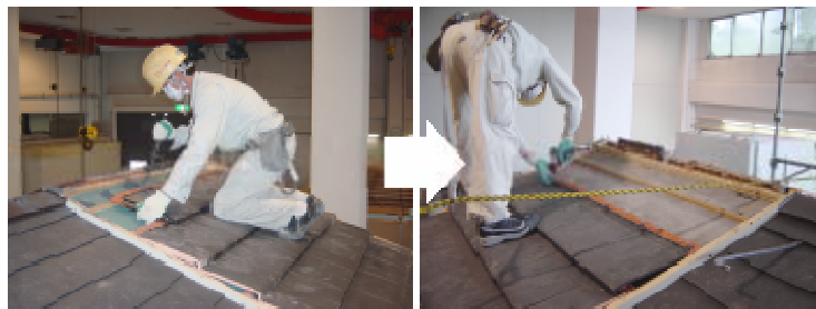
Photo 14 Roofing tiles removed. Right: “Improved”. Roofing tiles connected by wood screws can be easily removed without damaging the roof tiles.
