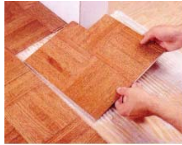
Figure 1. Installation of the flooring (Current design) – Floorings are nailed and glued to the floor sheathing.
