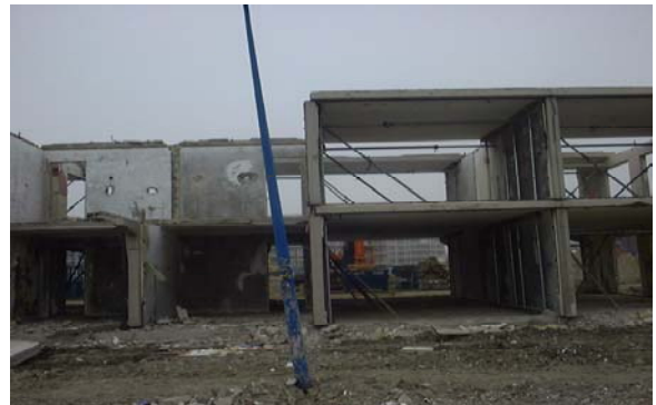
Fig5: After removing the floor it is clearly to see that the wall is not standing 90°. This will be fixed during construction
