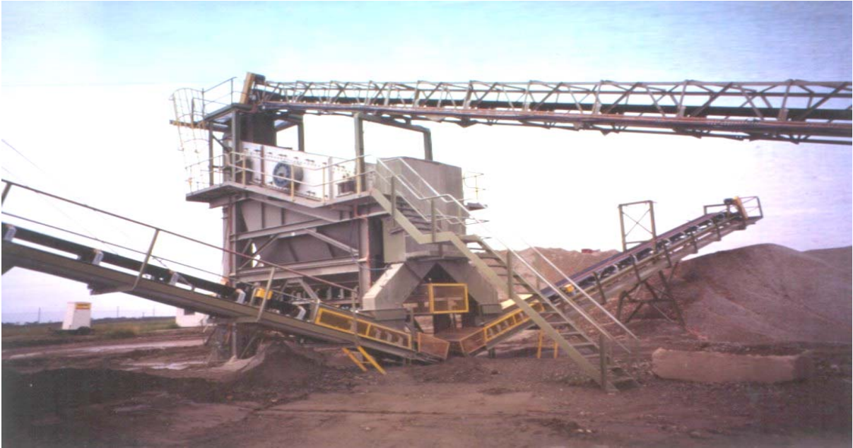
Figure 2 Concrete recycling plant, Brisbane.
