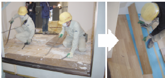
Photo 12 Hard wood floorings removed. Right: "Improved". Flooring can be easily removed without damaging the floor sheathings and floorings.
