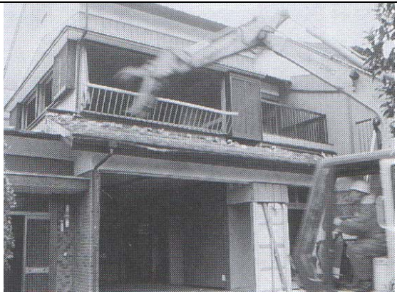
After removing tatami mats, doors, windows, and roof tile, start mechanical demolition.
