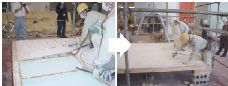
Photo 15 Floor sheathing removed. Right: “Improved”. Floor sheathings can be easily removed when they are not glued to the floor joists and connected by wood screw.
