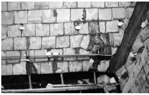
A typical example of the deterioration in the church roof as of 2000
