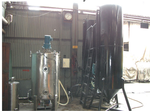
Fig. 4: Biodiesel pilot-plant 2,000 l/d (Semi-continuous batch type)
