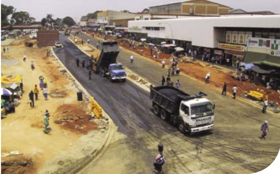
Construction of the Rautenbach / Watt / Roosevelt Link Road which forms part of the Alexandra Renewal Project.
