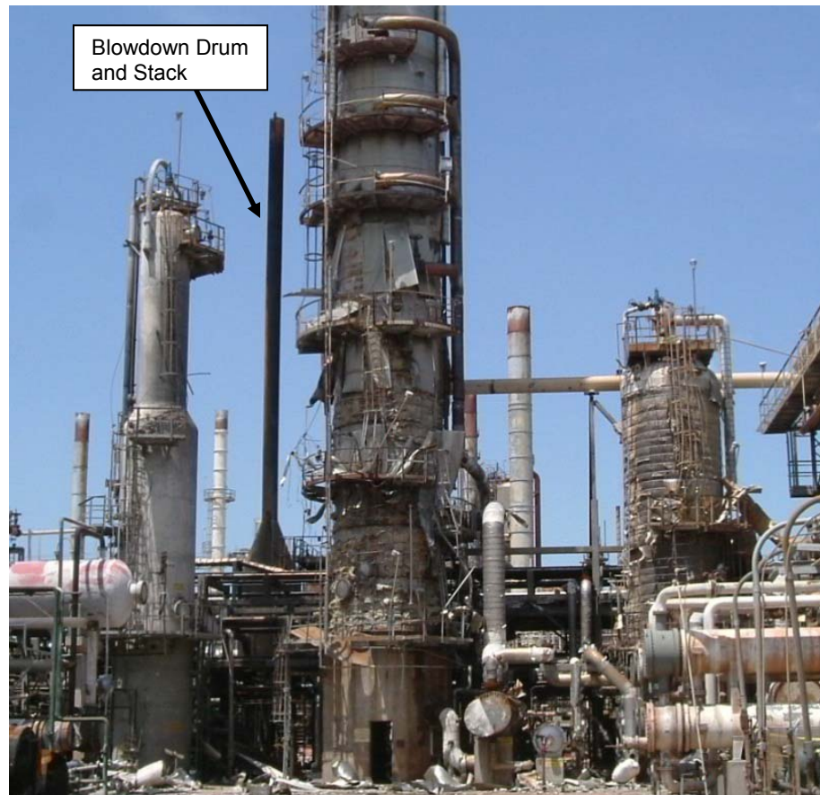
Figure 2-2 Blowdown Drum and ISOM Unit, After the Incident
