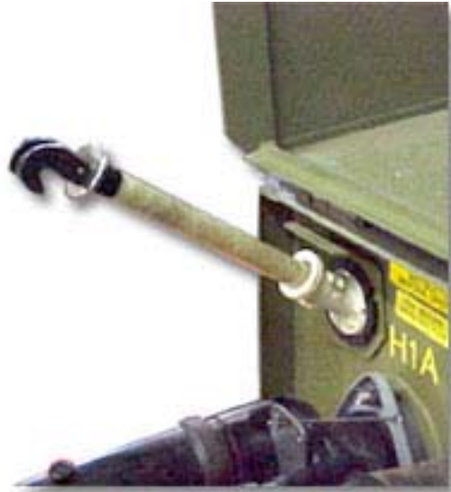
Figure 5: Bayonet Fuse in Padmounted Transformer
