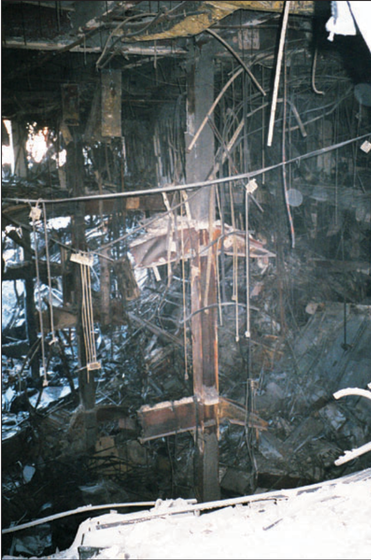
Figure 4-19 Internal collapsed area in WTC 5.
