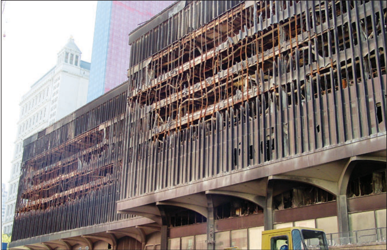
Figure 4-11 WTC 5 façade damage.
