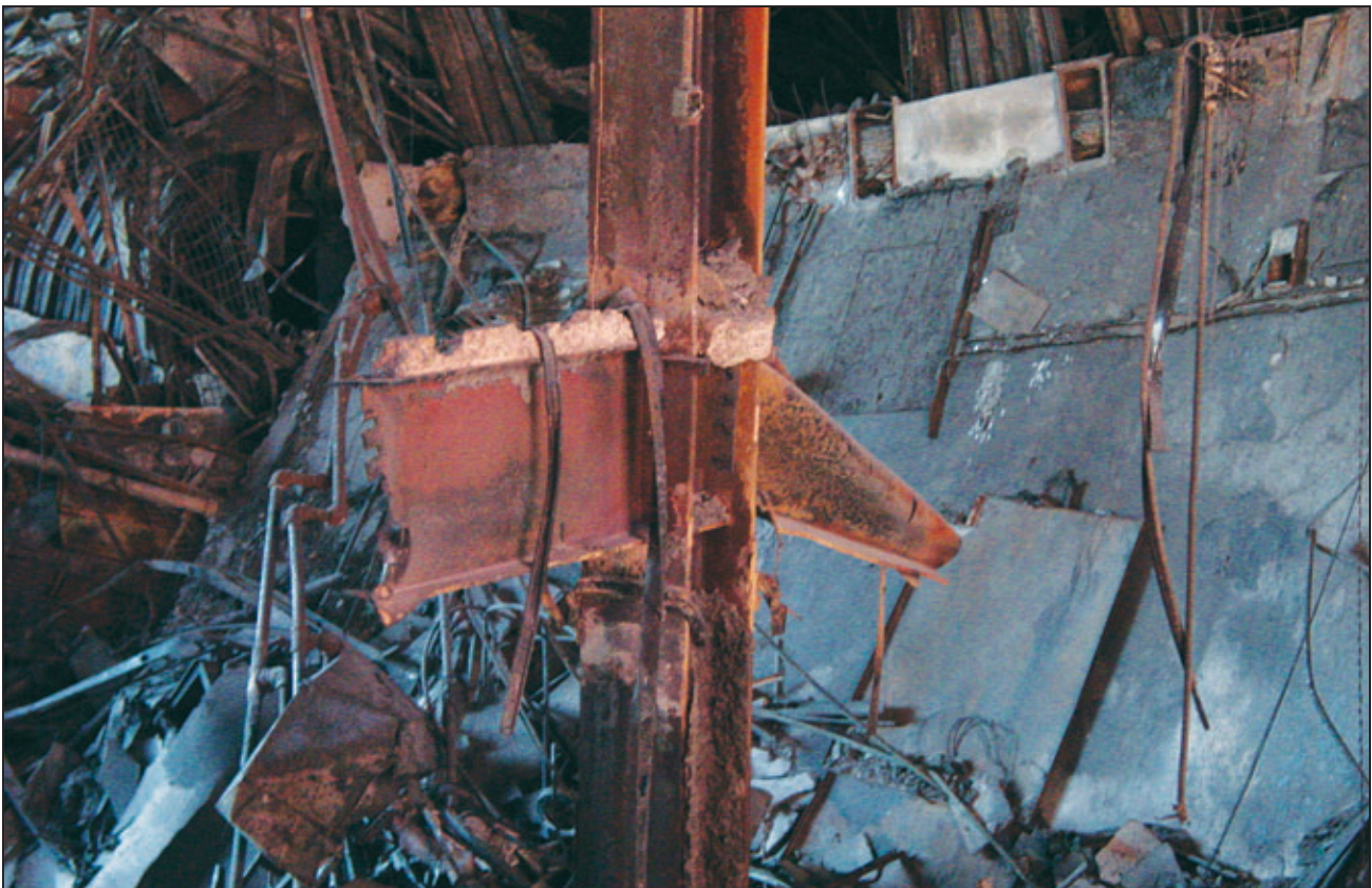
Figure 4-21 Internal collapsed area in WTC 5 with closeup of connection failure at column tree.
