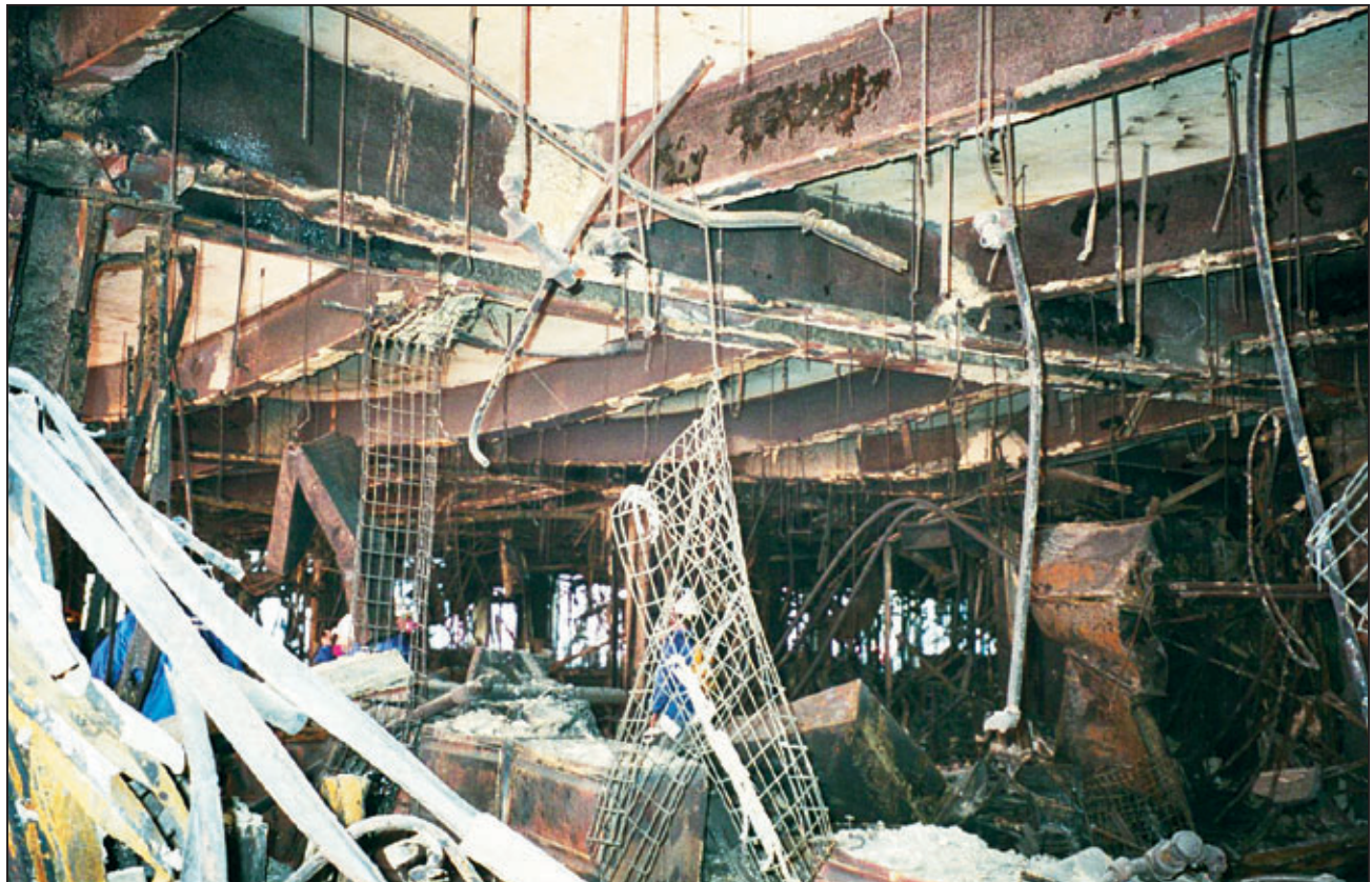
Figure 4-14 Deformed beams in WTC 5.
