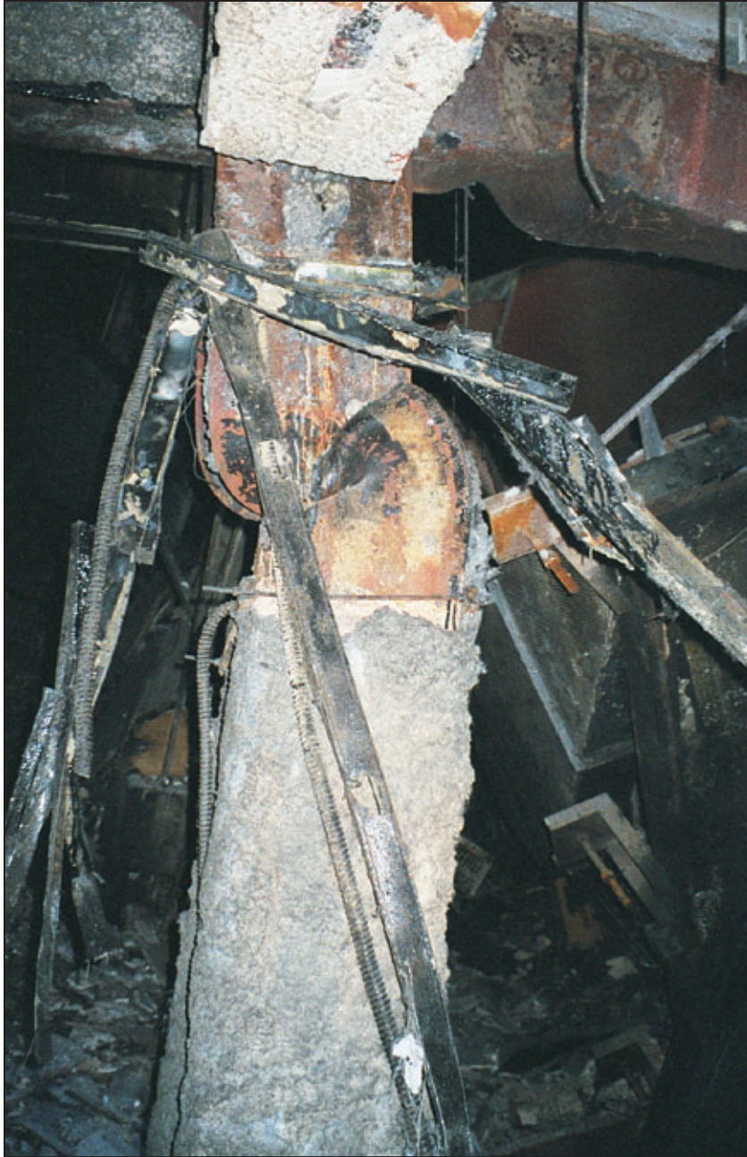
Figure 4-17 Buckled beam flange and column on the 8th floor of WTC 5 that was weakened by fire.
