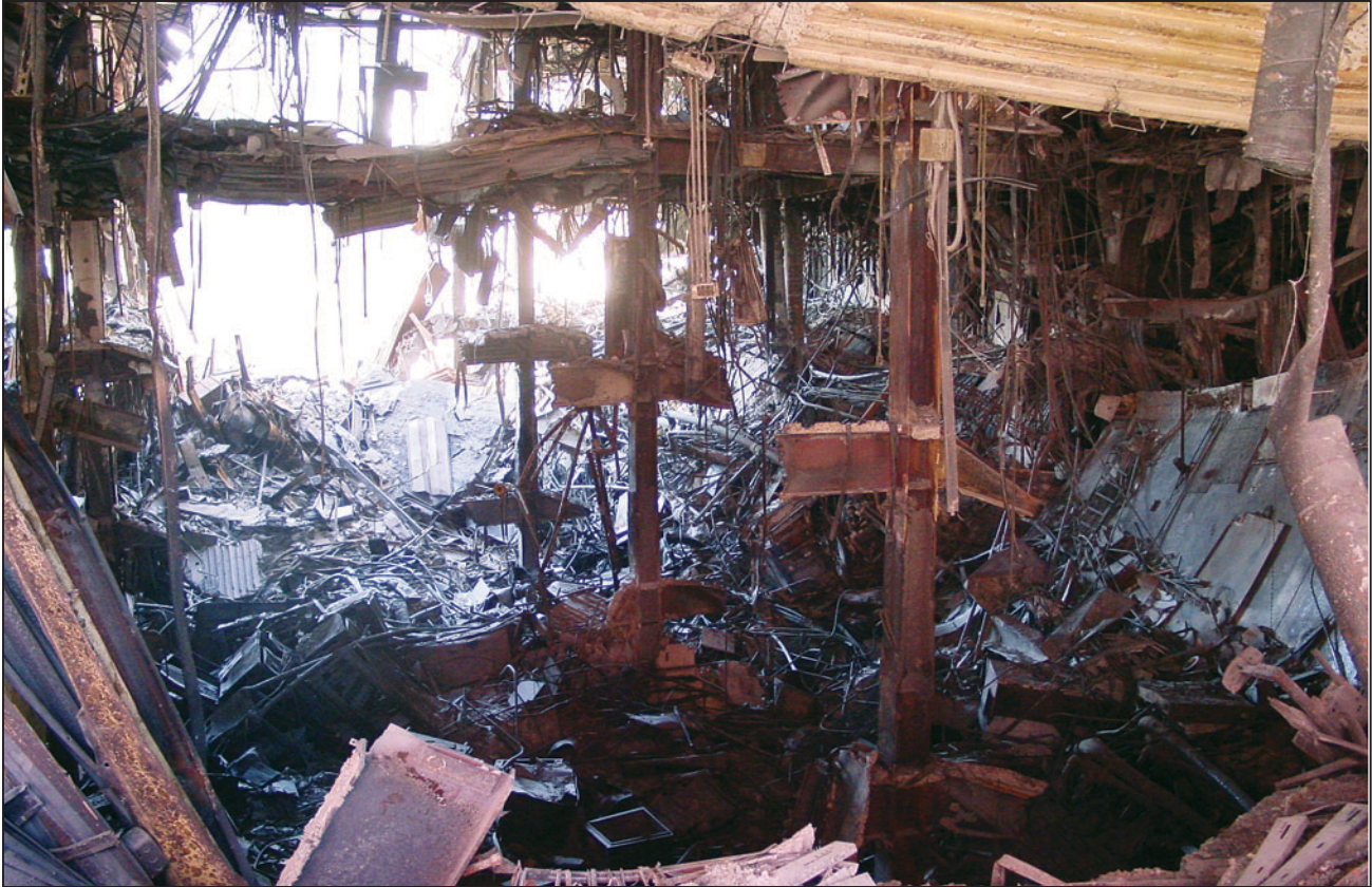
Figure 4-20 Internal collapsed area in WTC 5.
