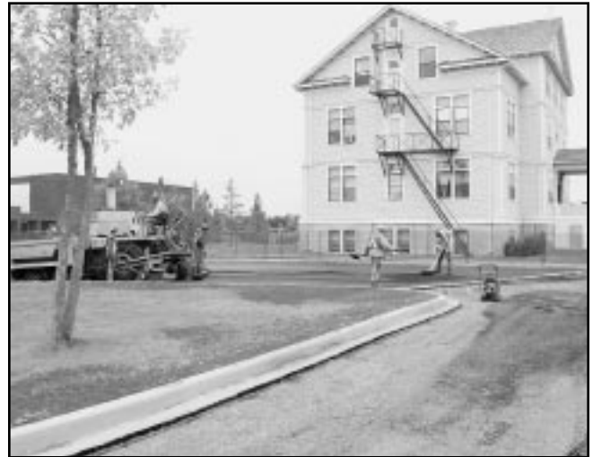
The lane outside Founders' Hall has pavement, curbs and sidewalks thanks to donations by Branco Concrete, of Wetaskiwin, and Border Paving, of Camrose.
