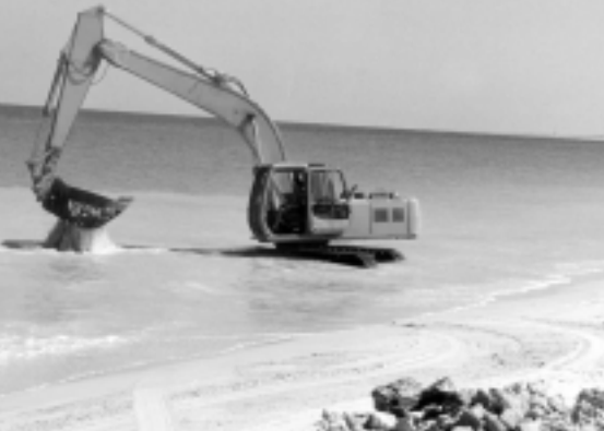
An excavator has been used to clear rocks from the Port Beach surfline.
