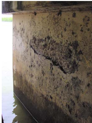
Figure IV Spalling of cover concrete at Southbound Pier No.5
