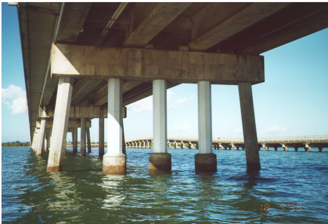
Figure VIII View of Concrete and Fibre Composite Encasement of Piles Houghton Highway Bridge Sandgate-Redcliffe
