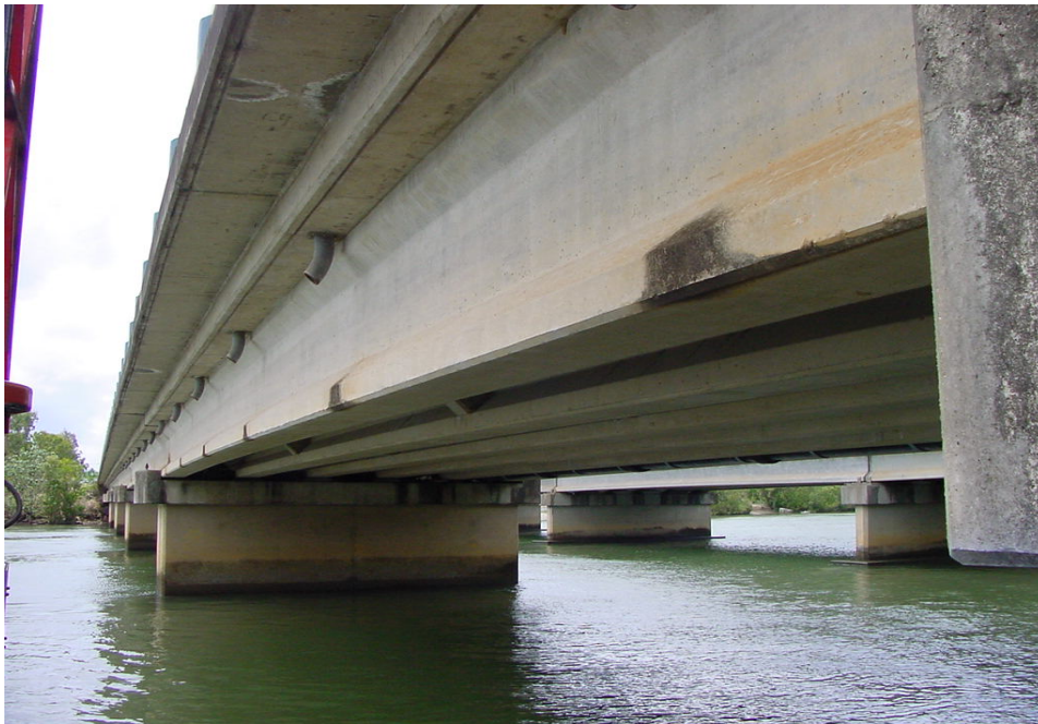
Figure I General view of Southbound Barron River Bridge at high tide note girders exhibit some alkali-silica reaction cracking under scuppers
