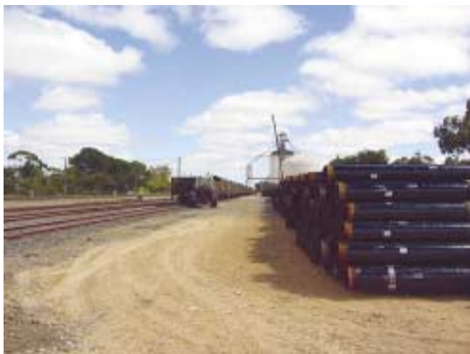
Lengths of gas pipe stockpiled at Tintinara in preparation for laying. (Photo 49042)
