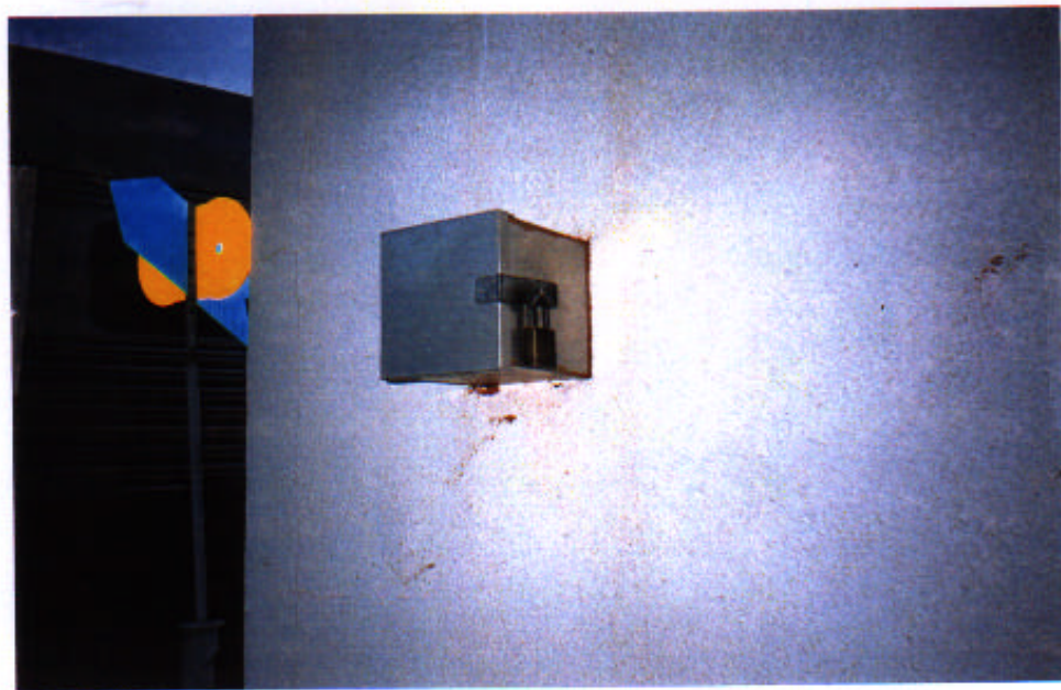
Figure 6: View of locked push button control box and yellow dumb bell indicating points set for loop
