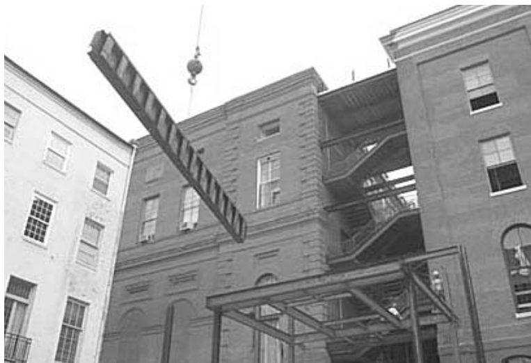
One of the massive steel beams of the Gallery Pavilion is set in place.
