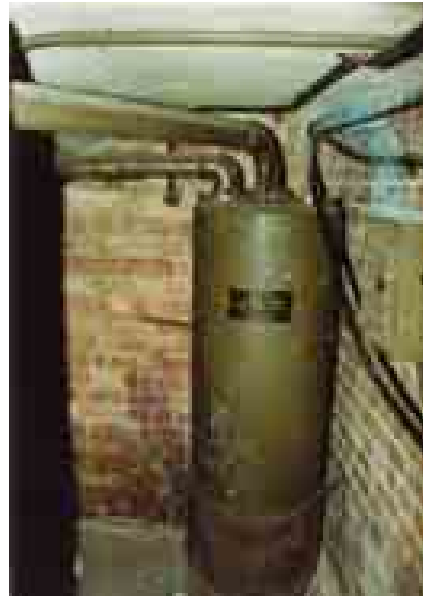
Fig. 40 The BVC centralised vacuum cleaner plant
