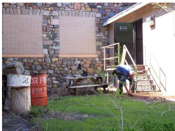
Facilities Manager Doyle Smith begins construction of the simunitions range that is inside building 6
