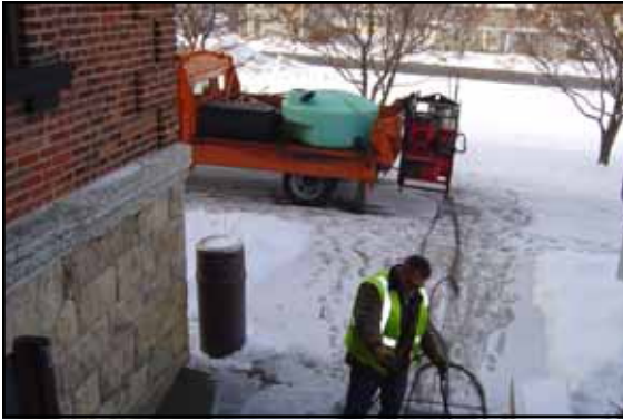
With little snow cover, one of our drains froze. Terry Hayner from the N. Shop worked all day to steam open the drain.
