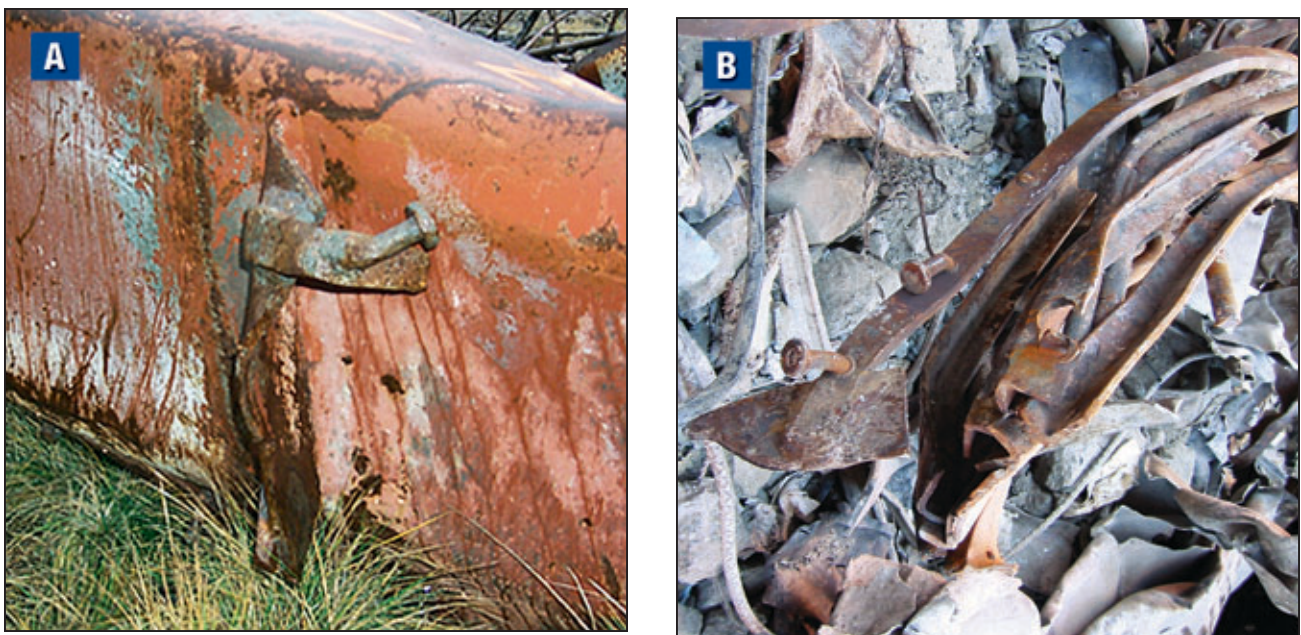
Figure B-10 (A) Bracket plate welded to the column/spandrel plate and (B) horizontal plate brace with shear connectors welded to the failed bracket.
