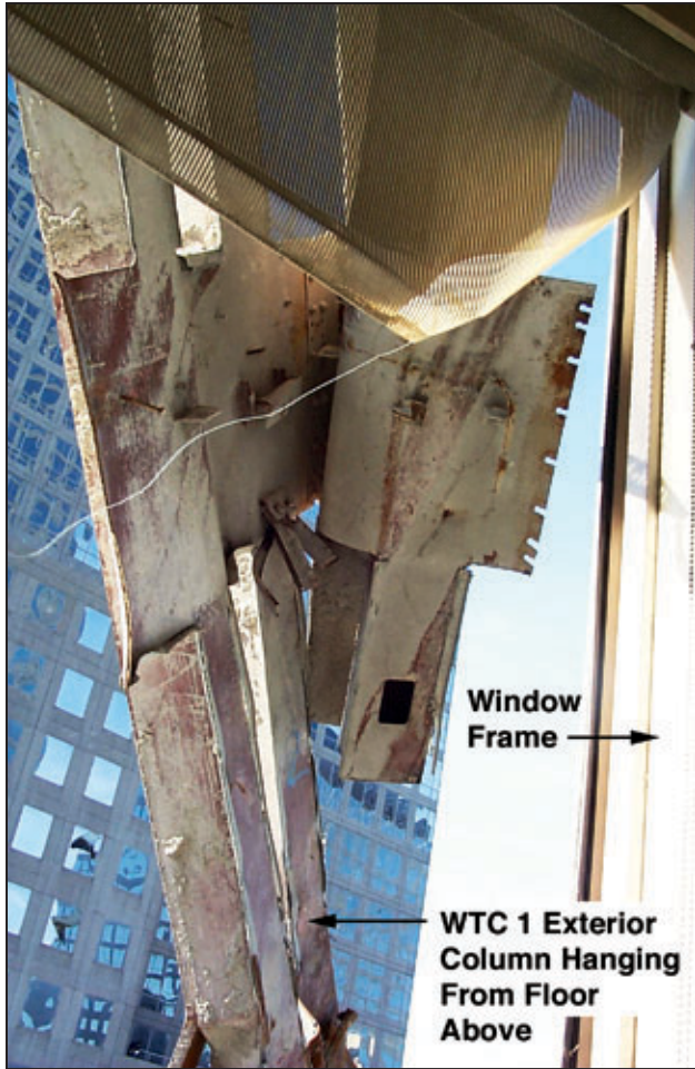
Figure B-5 Column tree showing bolt bearing shear failures of spandrel connection.
