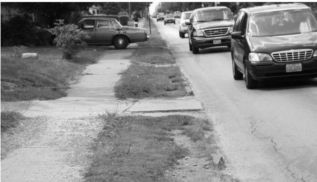
Example of sidewalk and curb in disrepair on Hudson Street.
