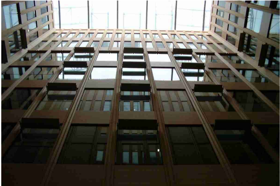
Figure 9: Picture of the completed inner courtyard , view from the ground level to the roof
