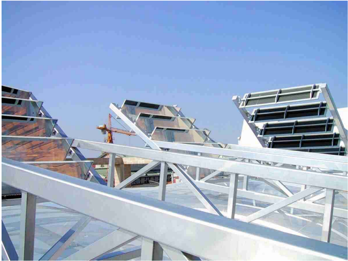
Figure 11: Picture of the redirecting mirrors installed on the roof
